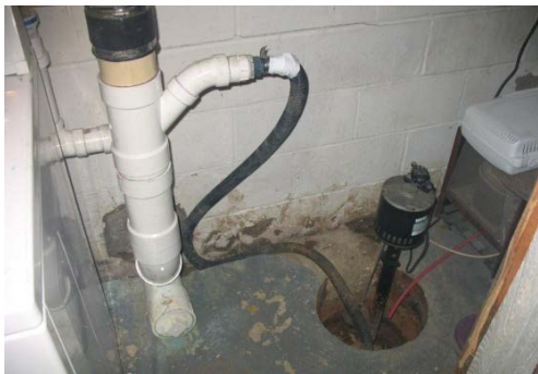
Private Source Inflow from a Sump Pump
