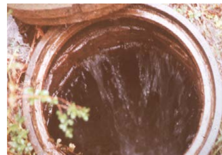
Inflow into a Manhole During Flooding
