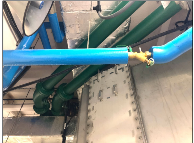
Ejection Piping (in green) in Odor Control Room
