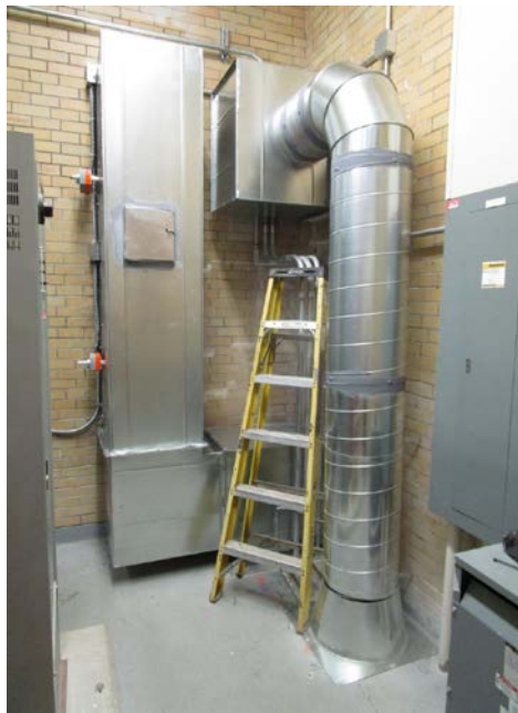
New Dehumidification Ductwork
