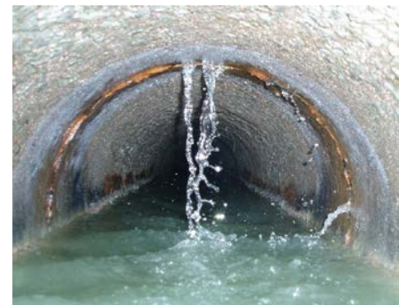
Infiltration into a Sanitary Sewer
